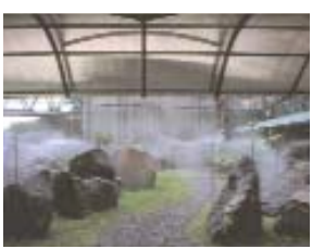
The misting-cooling system in the courtyard is activated for ten seconds every ten minutes during the dry season. The courtyard air flows into the building, providing humidity and cooling.
