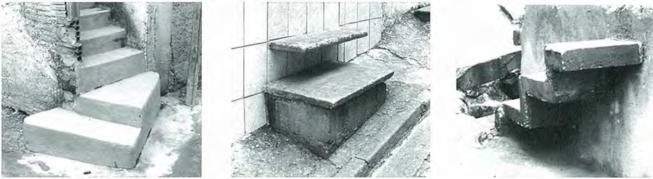
FIGURE 13. (LEFT) Landing step encroaching into an auto-accessible alley in São Remo.
