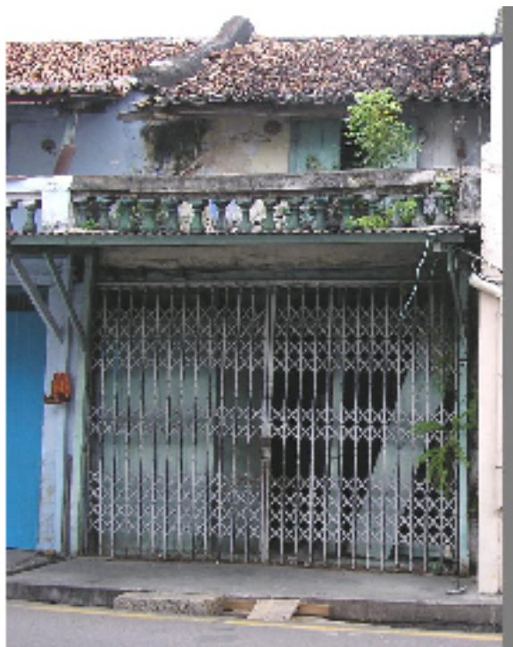
(Fig. 6). Dilapidated oldshophouse. Shophouse delapidado.
